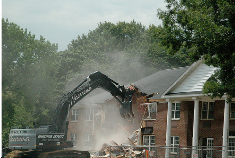
An interesting juxtaposition: Redevelopment of Governors Island in progress. Seems you can't escape construction no matter where you go...
